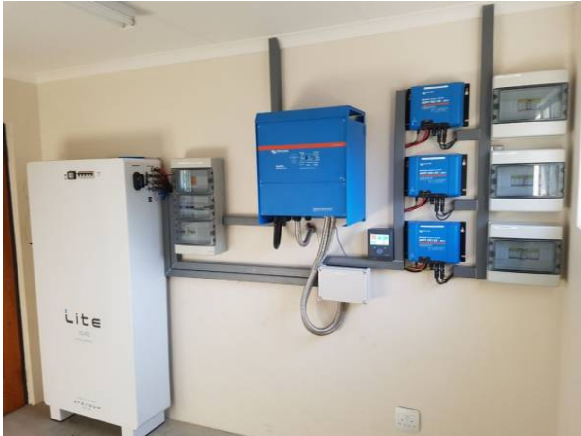
Figure 1 Typical Installation: Freedom Lite 60/42 with Victron 15kVA Quattro and 3x Ve Direct MPPT's
