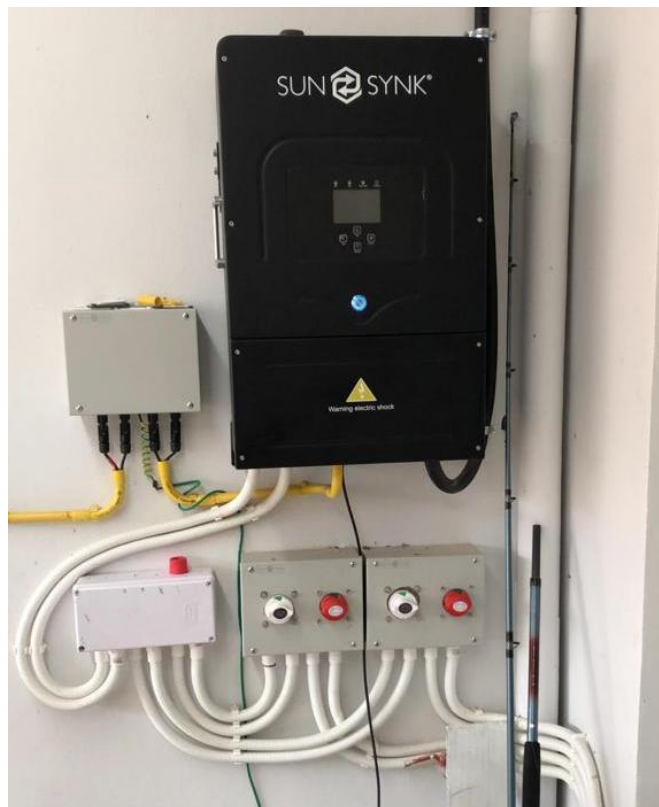
Figure 14 - Sunsynk inverter installation - black version.
