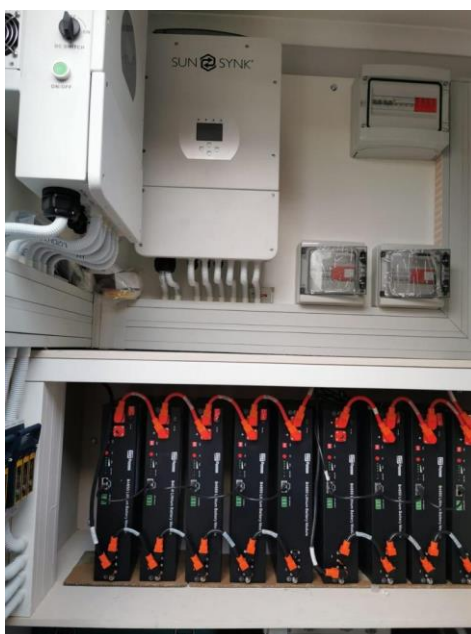
Figure 16 - Inverters with appropriate battery connections.
