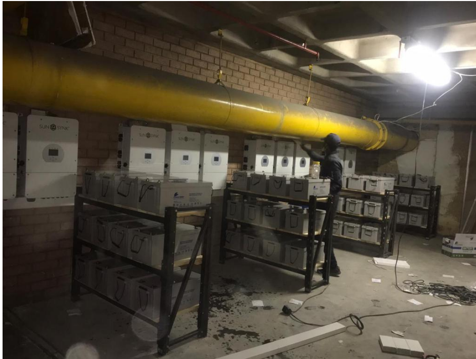
Figure 59 - Inverter installed in a dusty environment.
