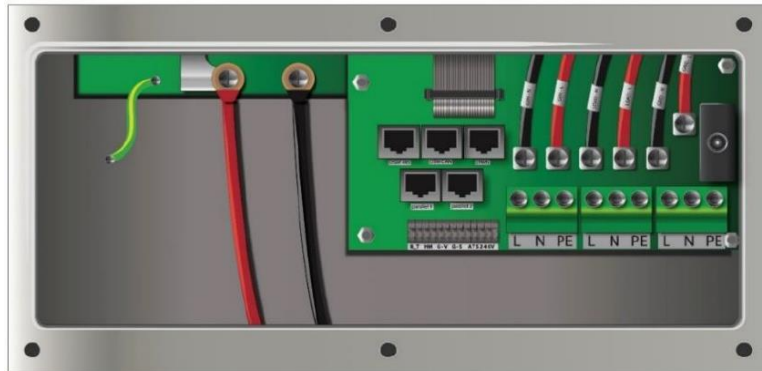
Battery connection of the 5kW model
