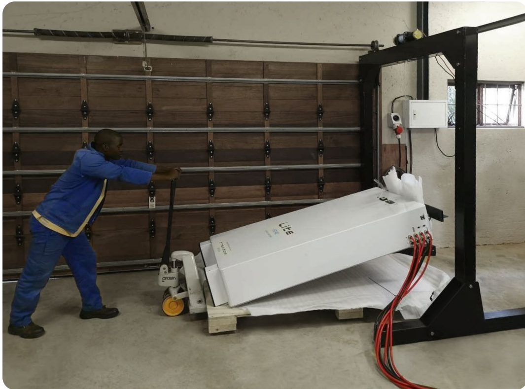
Fig 3.5 Site Assembled Gantry with Electric Hoist
